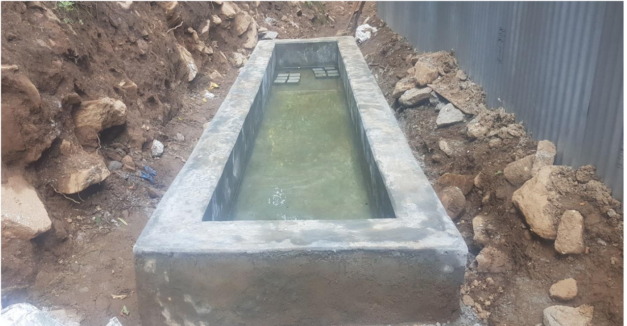
Figure 11: Cube curing pond at concrete lab.
