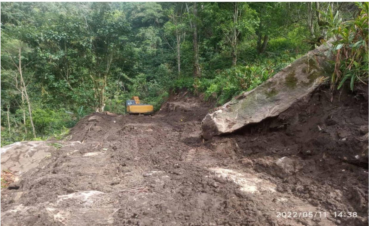
Figure 26: Excess road from powerhouse to surge tank
