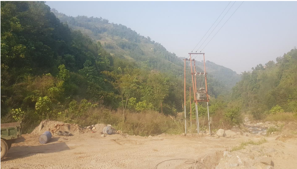
Figure 16: Transformer for construction power
